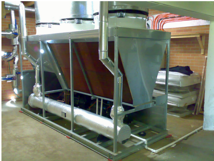
220kW chiller for The Coast Golf Club involved customisations like copper/copper condensers, hot dipped galvanized frames and stainless steel panels to withstand the harsh coastal environment
